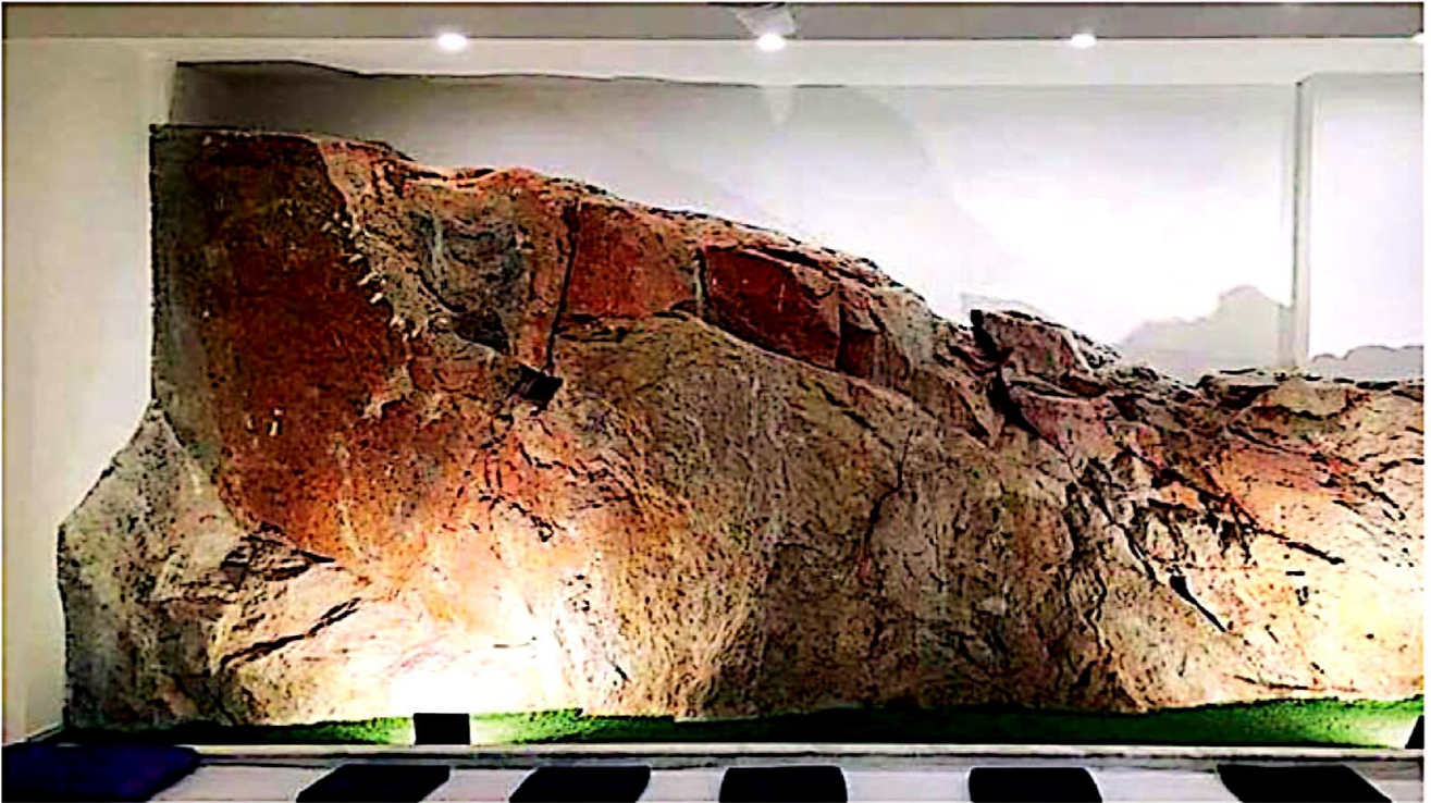
The conversational piece of the building is certainly the existing rock being retained as a wall and also forming part of the building foundation.
